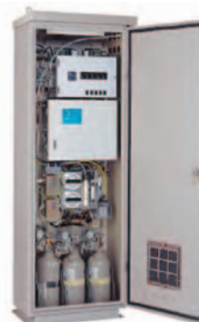
Continuous Emission Stack Gas Monitoring System
